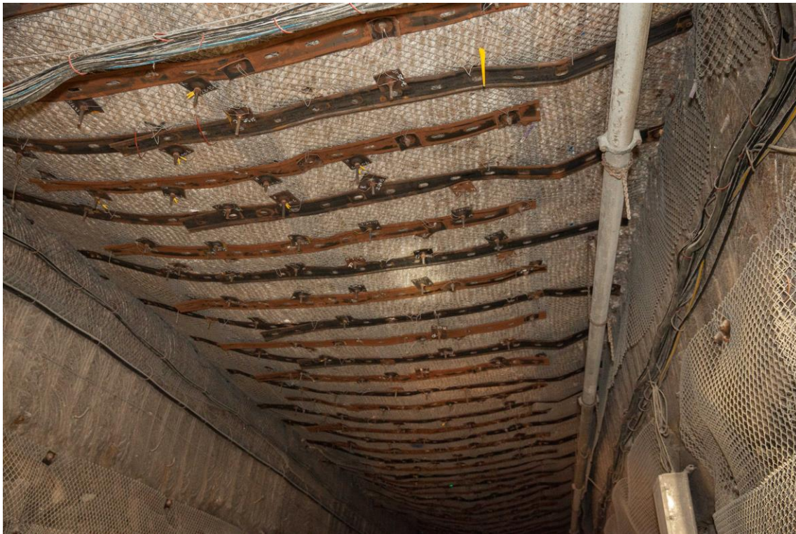
Figure 4: Bolts within the repository to slow salt displacement rate
